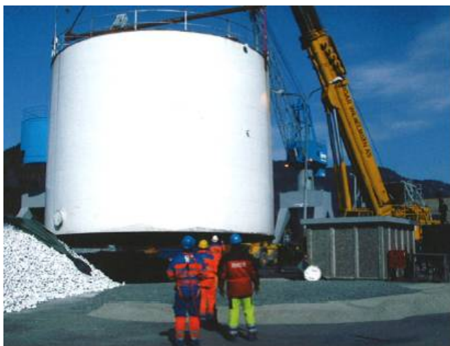
Figur: Lagertank for Dustex monteres i Orkanger
